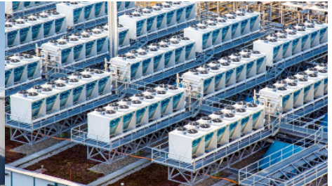
HVAC / Air Conditioning Systems
